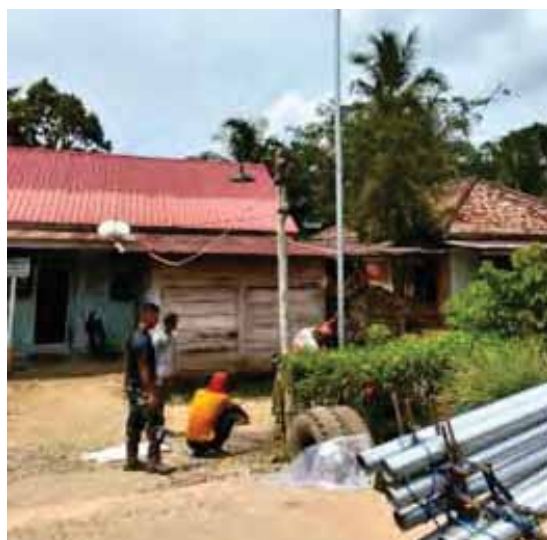
Pemasangan lamput jalan bertenaga surya di Desa Beringin Makmur II, Desa Simpang Tebing, Desa Bumi Makmur, dan Desa Sumber Sari Installation of solar-powered streetlight at Beringin Makmur II Village, Simpang Tebing Village, Bumi Makmur Village and Sumber Sari Village
